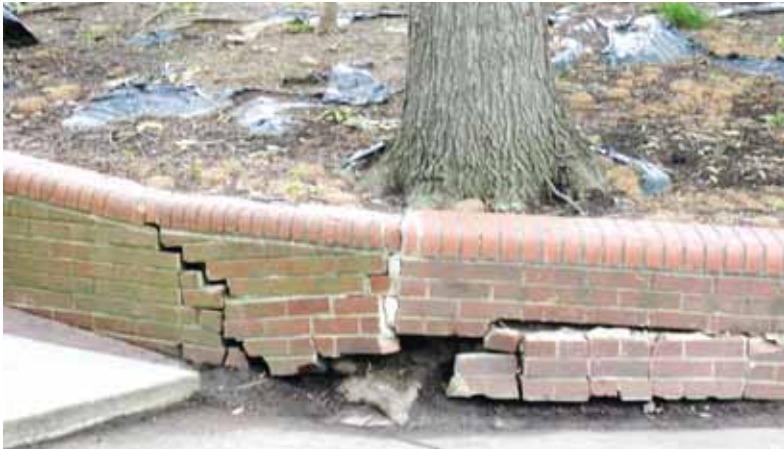
Some of the retaining walls in Town Center West Park are unstable.
